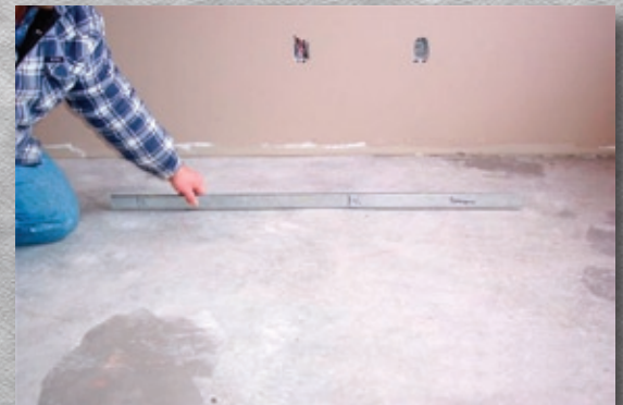
An example of a wavy concrete surface
