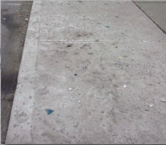
Light scaling of a concrete sidewalk
