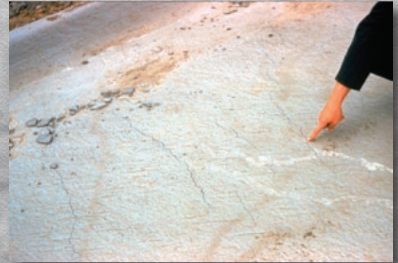
Plastic shrinkage cracks on exterior flatwork
