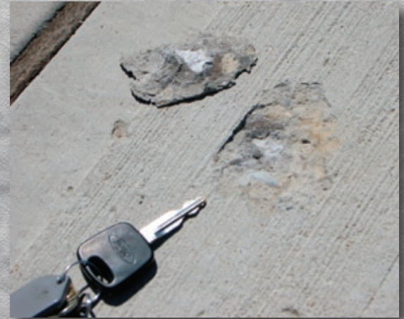
Popout surface damage caused by the fracture of a soft aggregate particle during winter freeze/thaw cycles
