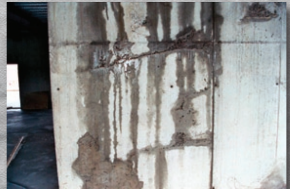
Honeycombing in a residential shear wall
