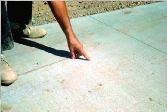
Crazing on exterior flatwork
