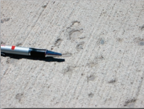
Mortar flaking on a concrete sidewalk – Note that the aggregate is sound and only the mortar above the aggregate has failed
