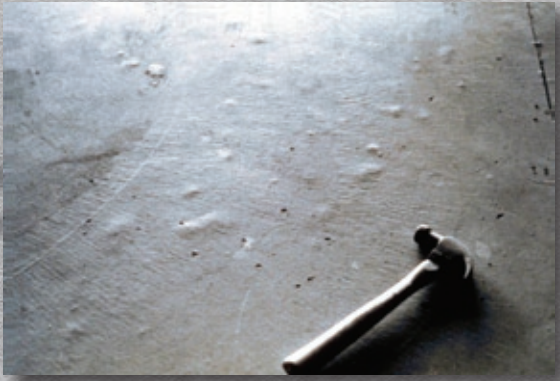
Blistering concrete surface
