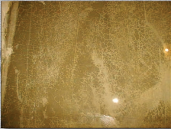
Crazing on a residential garage floor slab
