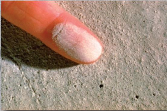
An example of a dusting concrete surface
