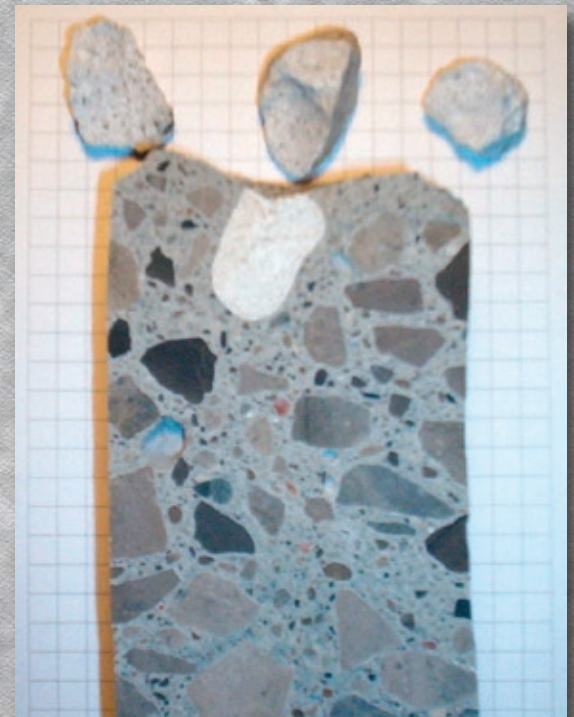
A cross-sectional view of a concrete core taken from a popout area – note the large chert particle in this limestone aggregate source that is responsible for the popout
