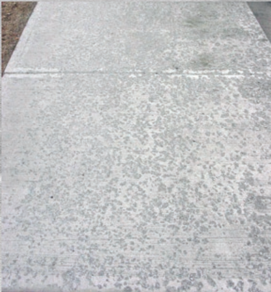
Medium scaling of a concrete sidewalk
