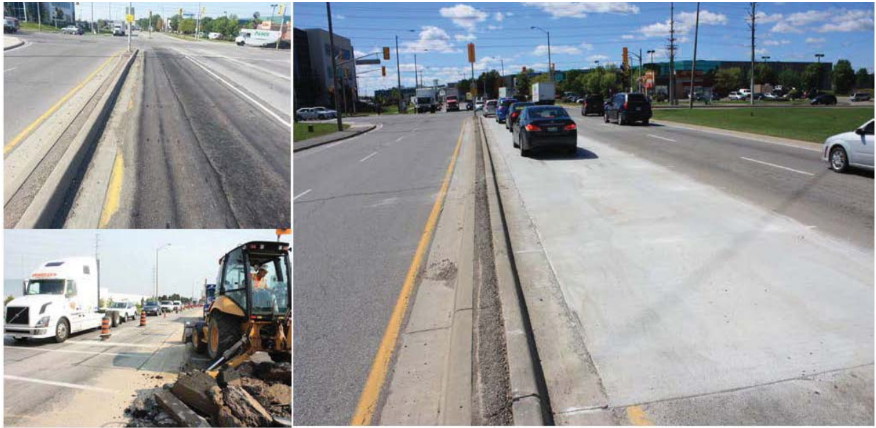
Figure 5.1 – Asphalt rutting and concrete left-turn lane installation in Mississauga (provided by Concrete Ontario).
