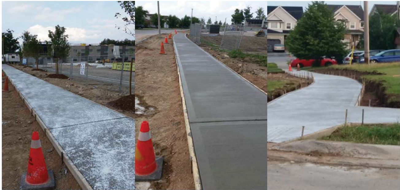
Figure 15.3 – (Left / middle) Insufficient curing examples and (right) adequate curing compound application (provided by Concrete Ontario).
