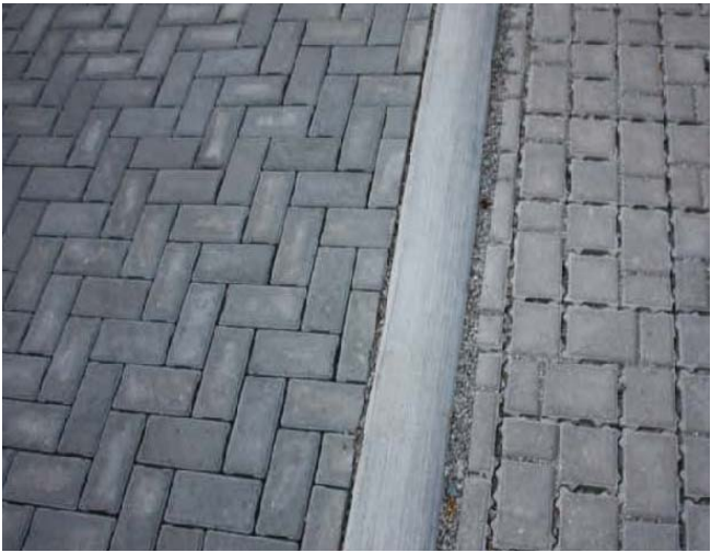
Figure 3.7 - Interlocking Concrete Pavers (ICP) for a Permeable Pavement Application (provided by Concrete Ontario)
