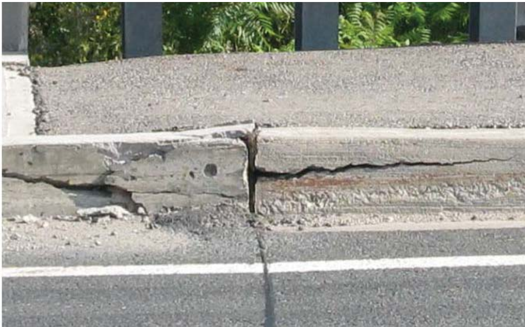
Figure 9.7 - Joint failure due to expansion (provided by County of Essex)
