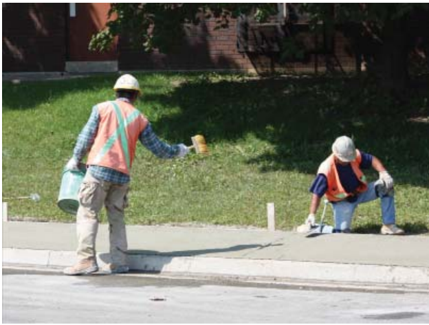
Figure 14.4: Concrete finishing bad practice (provided by Concrete Ontario)
