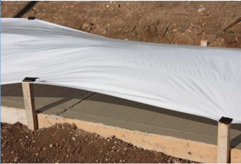
Figure 15.2: Unsecured protection system (provided by Concrete Ontario)
