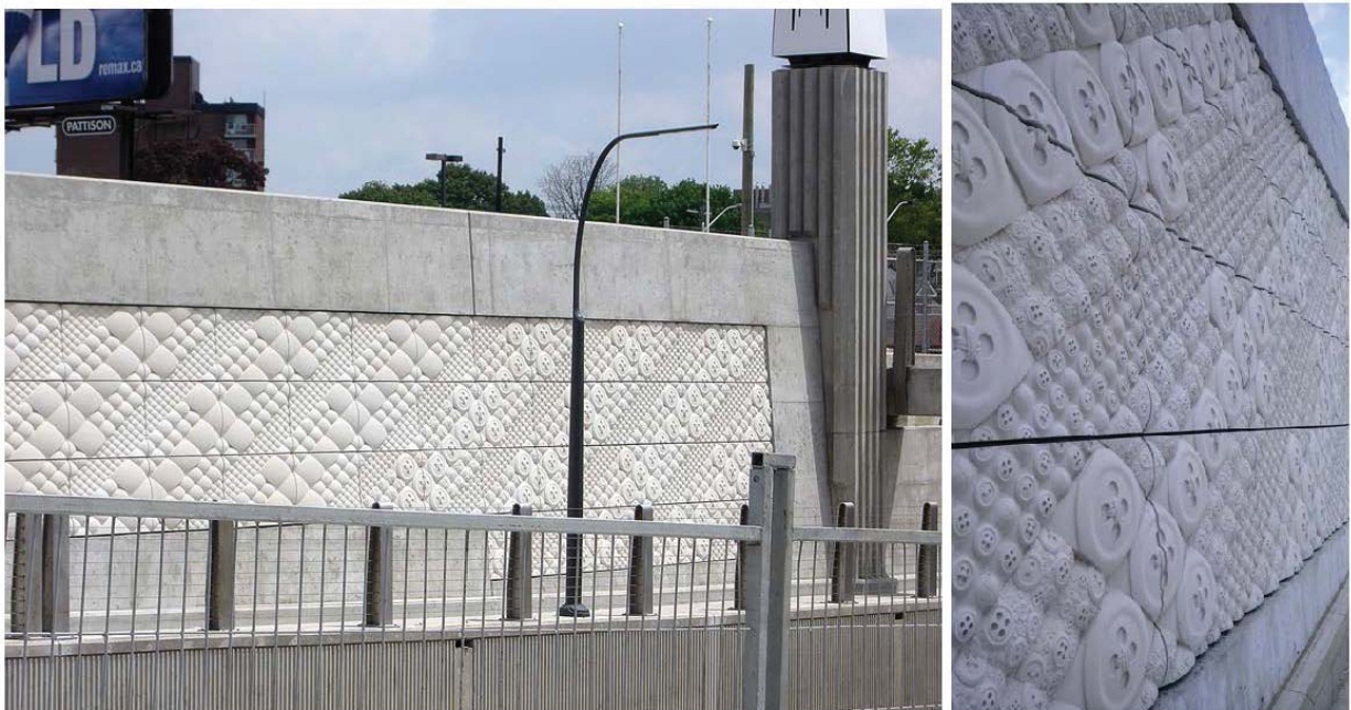
Figure 8.2 – Architectural precast concrete bridge abutment, City of Kitchener (provided by Region of Waterloo).
