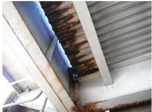
Figure 4.3 - Below-deck inspection and steel corrosion deficiency
