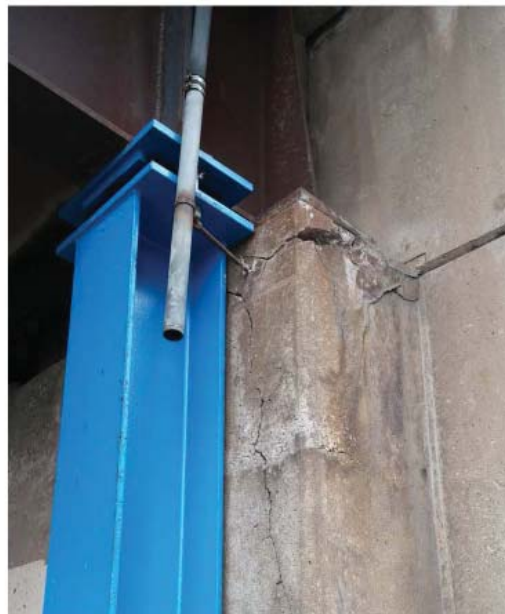
Figure 4.4 - Bearing seat spalling and temporary support installation
