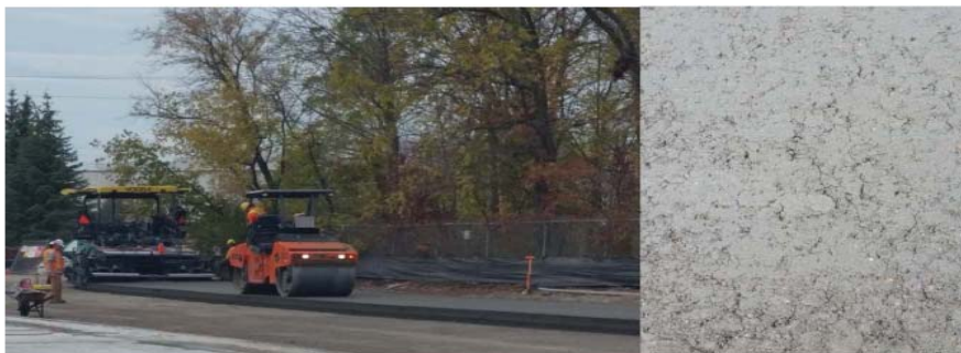
Figure 3.5 - Roller Compacted Concrete (RCC) for an industrial facility (provided by Concrete Ontario).
